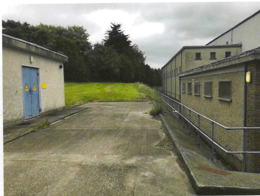
Image 5 The MV building on the left, and the control room building on the right, with the taller 38kV station building immediately to the rear and the dominant 110kV building in the background
