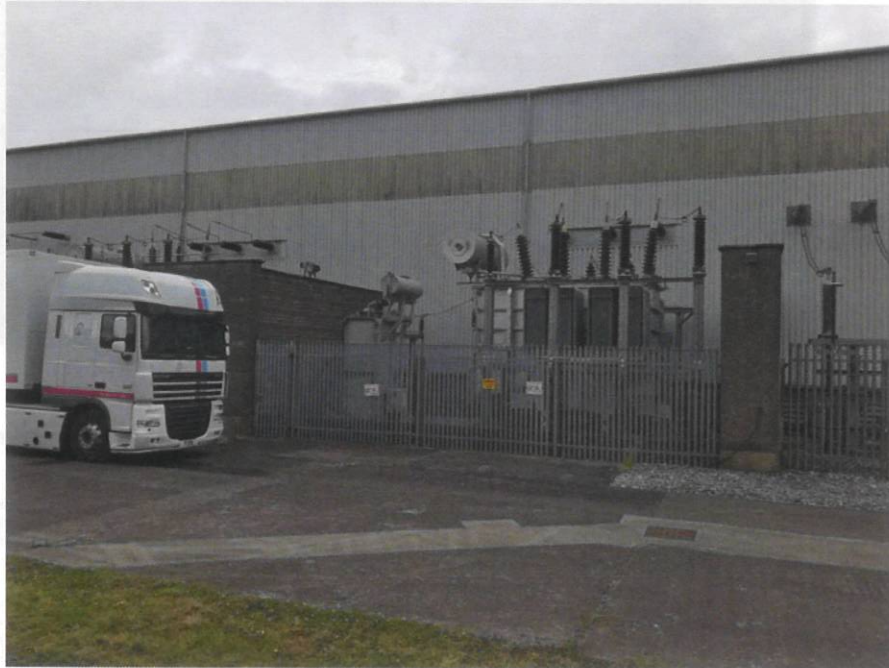
Image 6 Outdoor electrical plant (transformers) located along the southern elevation of the existing 110kV substation building
