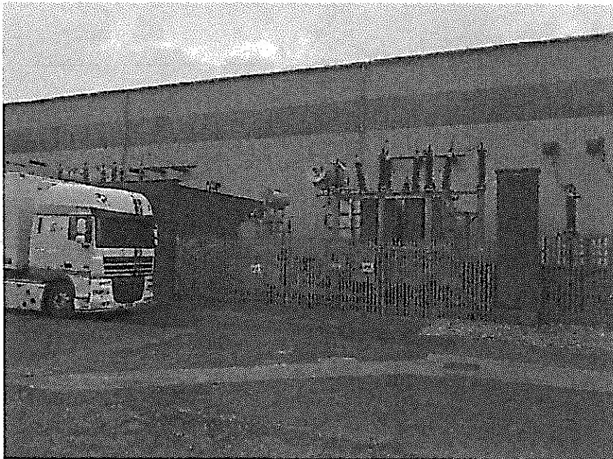
Image 6 Outdoor electrical plant (transformers) located along the southern elevation of the existing 110kV substation building
