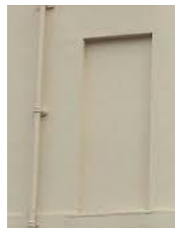
New masonry elements in / on existing structures shall be set back 30-40mm so that the original and new structure can be read separately.
