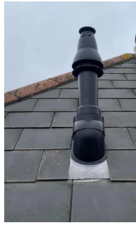
Example of boiler flue in slate roof with lead flashing.
