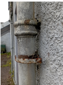
Existing profile detail on SVP to be simulated in proposed new SVP profiling.
