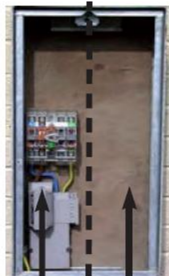
ESB Networks Equipment Customer Equipment
