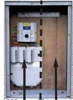
ESB Networks Equipment Customer Equipment
