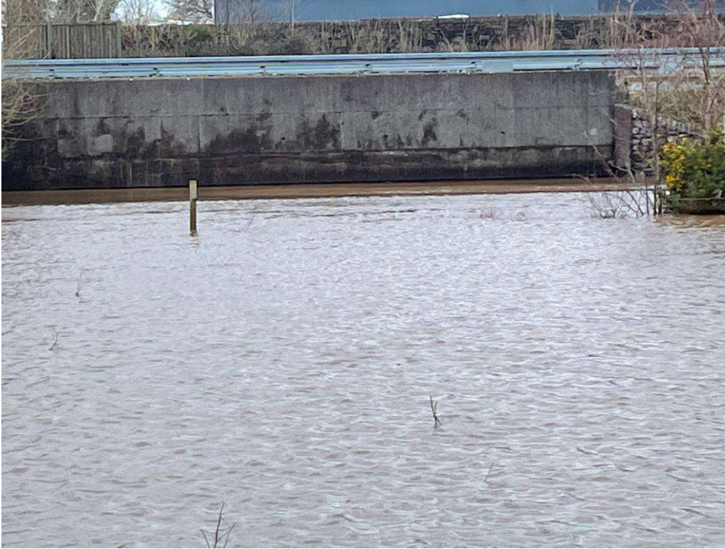
Photo 15: Maglin North Culvert under N22, just upstream of confluence with Maglin South
