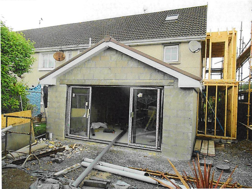
Rear elevation of house with single storey extension to the rear and side extension under construction
