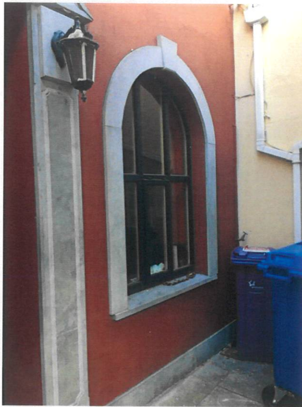
Image of existing window to side of bar door from inside Douglas Street gateway
