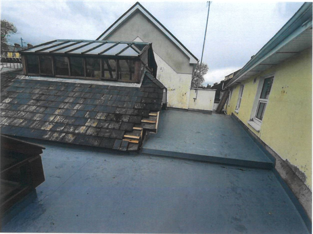
Roof image showing lantern rooflight to be removed to form open internal courtyard
