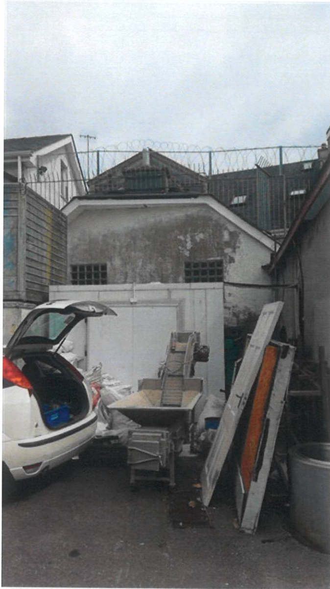
Image of rear elevation from private yard – note glass block windows as shown on rear elevation drawings
