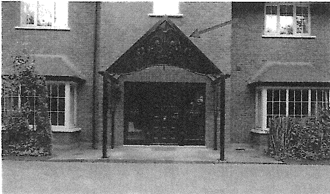
Part of subject dwelling to which works are proposed Canopy primarily finished in glass and supported with 2 no. metal supports to be amended to a flat roof fully enclosed porch, to include the bringing forward of the existing front door to serve the new enclosed porch
